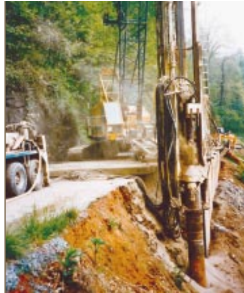
DR-24 mast kit mounted on crane leads to set foundation pilings for a retaining wall.
