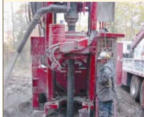
DR-24 shown in typical domestic waterwell application. Note the discharge swivel atop the casing which diverts the cuttings.
